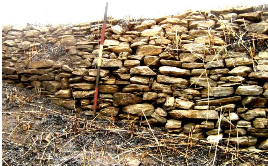
Fig. 10: A Terrace Wall (Photo by William N. Gblerkpor)
