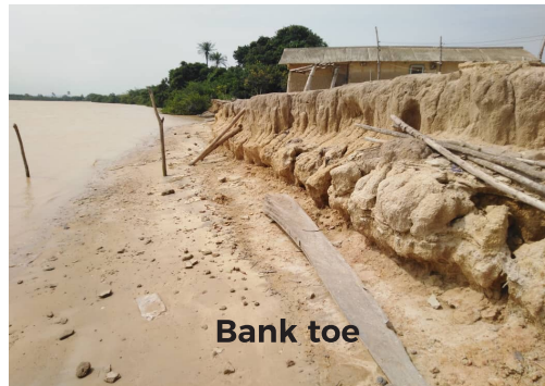
Fig. 2b: Building threatened by bank erosion at Krobo
