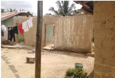
Fig. 3a: Collapsed building at Twansukoda in Twifo Praso
