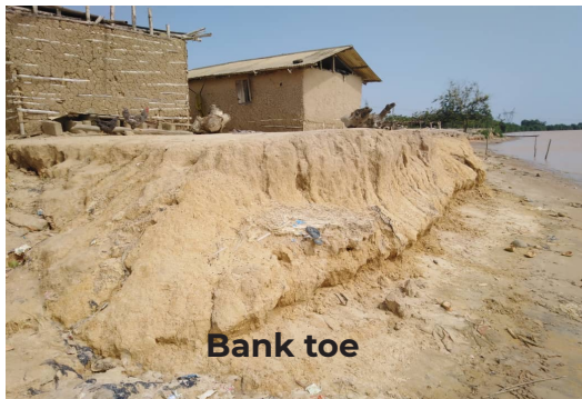
Fig. 2a: Buildings threatened by bank erosion at Bosomdo
